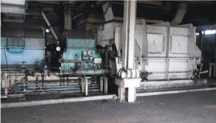
Figure 1. TTK 72 in. x 114 in. granulator installed at National Thermal Power Corp. Ltd in Barh, India.
